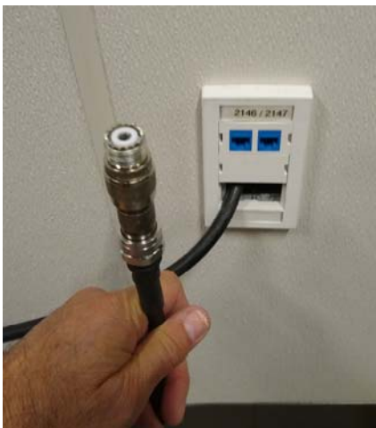
CC-6 – Antenna Connection
