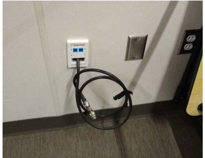
CC-5 – Antenna hangs from outlet
