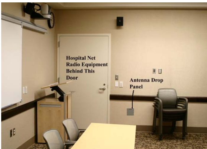
Figure 9: Radio Equipment Door and Antenna Drop Panel in Conference Room A
