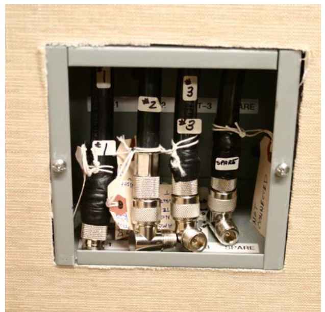
Figure 10: Antenna Drop Panel. Coax on the right is a spare and NOT connected to an antenna.
